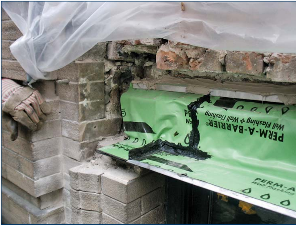
Figure 10 – Installation of flashing system, including end dam to protect underlying shelf angle at window head.
