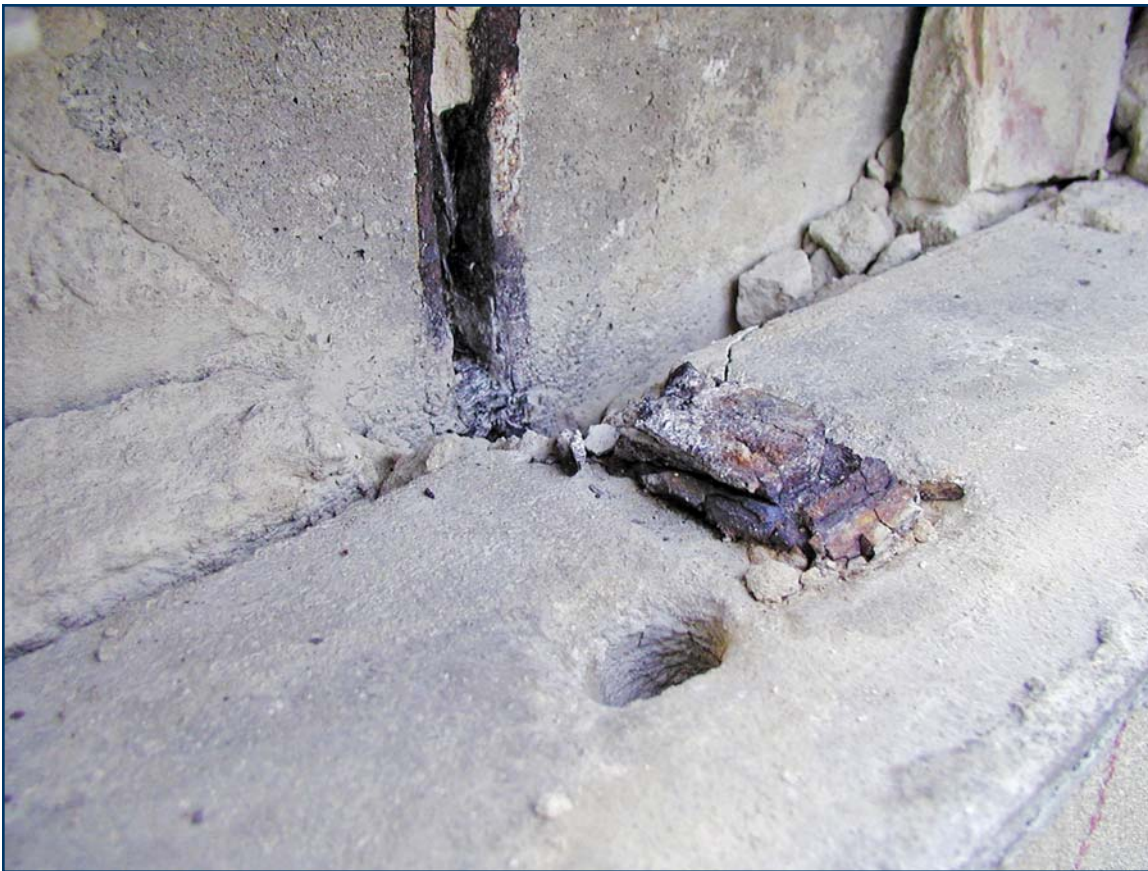
Figure 8 – Complete loss of lateral anchorage.
