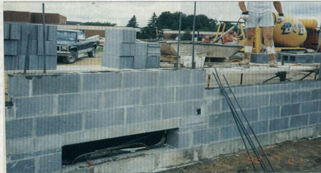
The plans call for continuous reinforcement 4 feet on center, which may not be practicable on walls with windows. Note how masons bent the rebar and changed spacing at openings.
